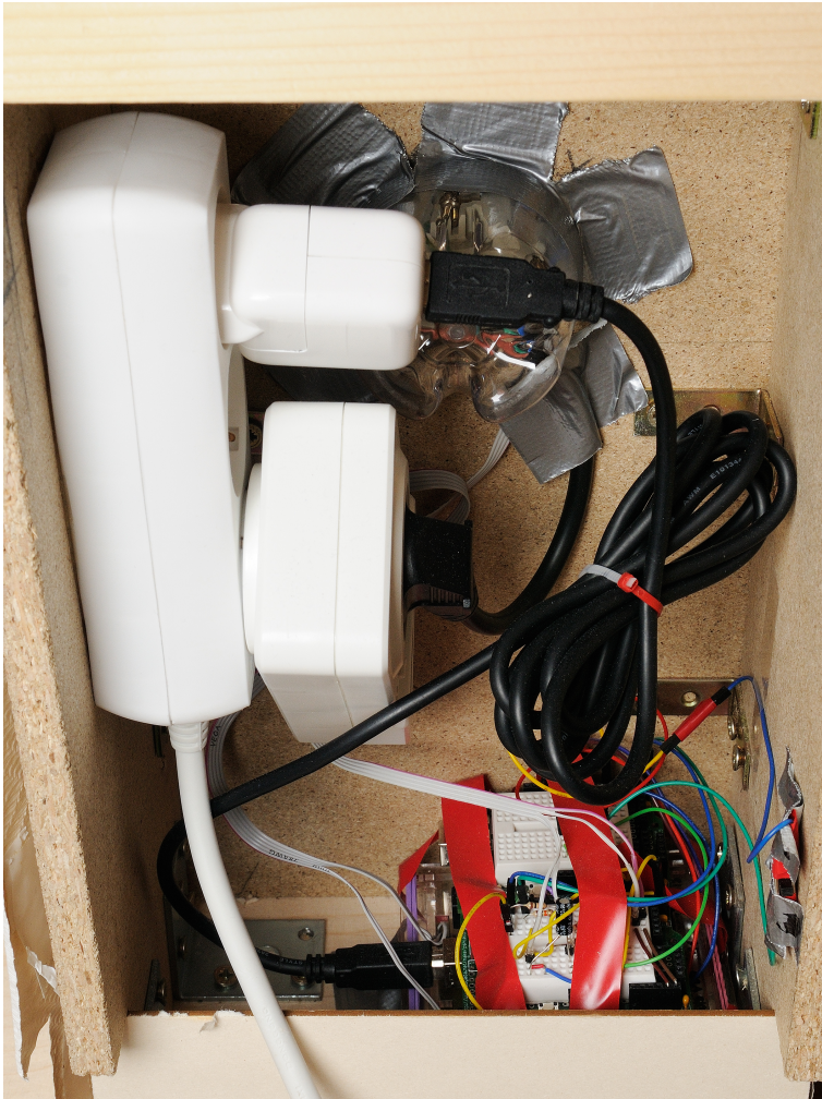
Figure 6.7: Backside of the Mock-Up Wall: Microcontrollers, Power Adapter, Modified Smart Meter, Extension Cord, and Wires
